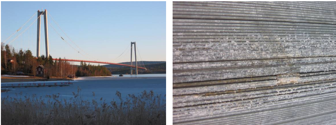
Figure 13 Högakusten Bridge, Cable works commenced and condition of wires on bottom of cable
