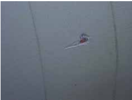
Figure 37 Puncture Requiring Cut Procedure
