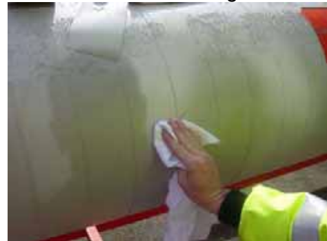
Figure 35 Clean Affected Area with Xylene
