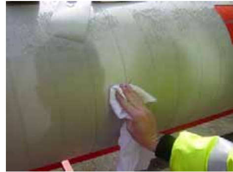
Figure 42 Clean Affected Area With Xylene
